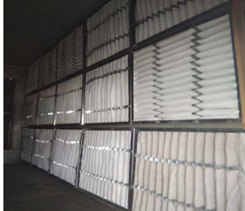
Enhanced air filtration and purification process with MERV 8 & 13 Filters
